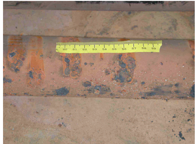
Figure 2. Pits and tubercles observed on failed boiler tube examined at the condominium. Note rusty streaks oriented at right angles to the tube length, which indicate active corrosion under stagnant conditions.
